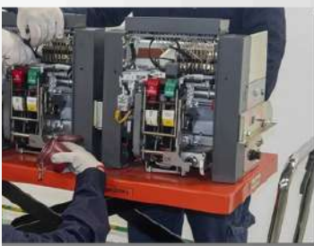
Circuit Breaker Maintenance & Testing
