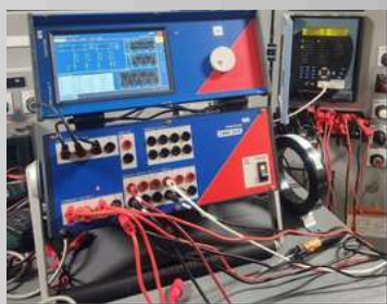
Protection Relay Testing
