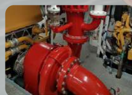
FIRE FIGHTING & WATER PUMPS
