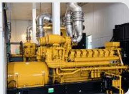
MAIN & AUXILIARY ENGINES
