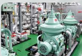
FUEL & LUBE OIL SEPARATORS
