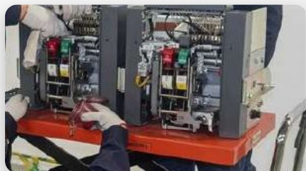
Circuit Breaker Maintenance & Testing
