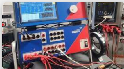
Protection Relay Testing
