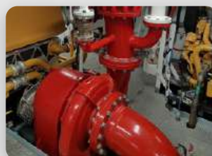
PUMPS & WATER SYSTEMS
