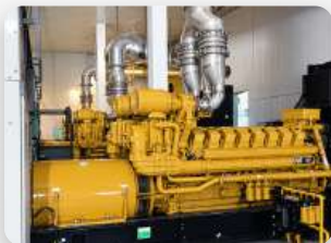
DIESEL ENGINES & GENERATOR SETS
